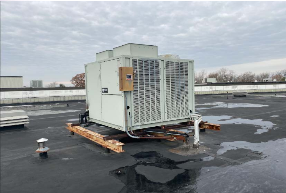
Existing Kitchen A/C Unit
