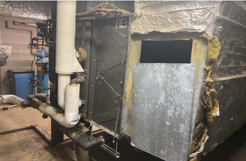
Existing Make-up Air Unit
