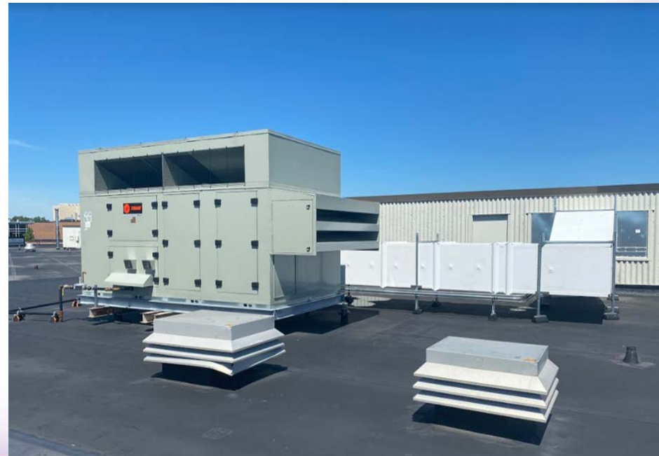
New Kitchen MUA Unit Installed
